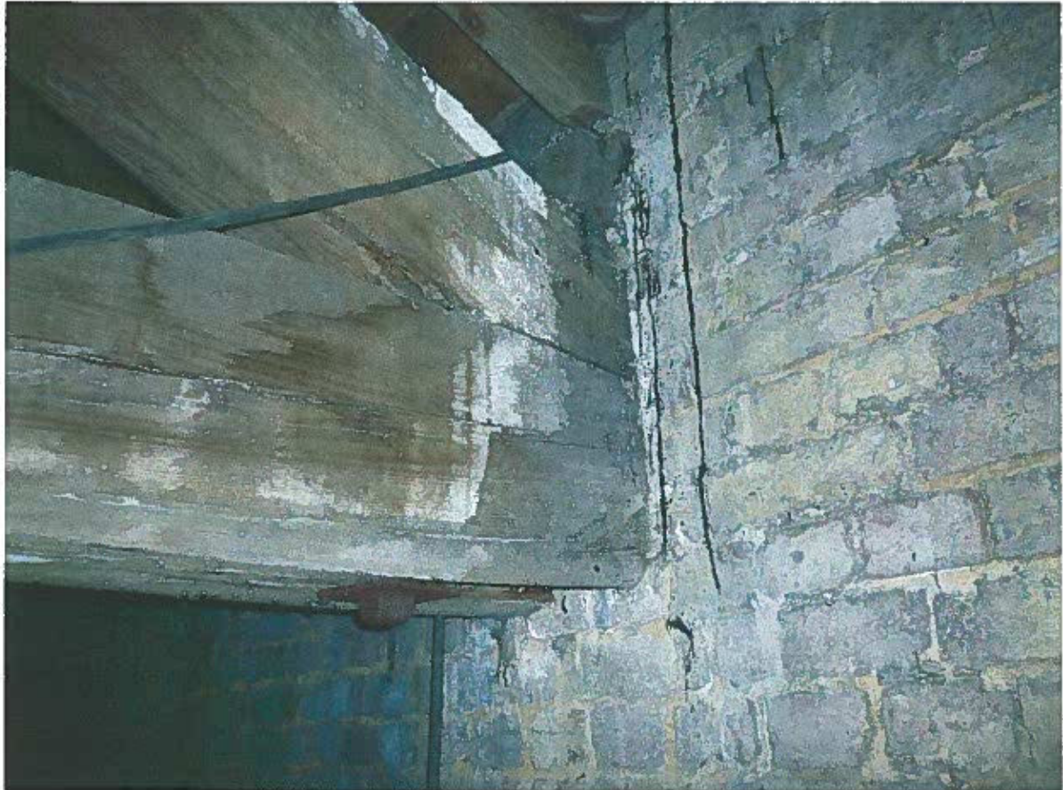
Picture 3 – Truss end suspected rotten
