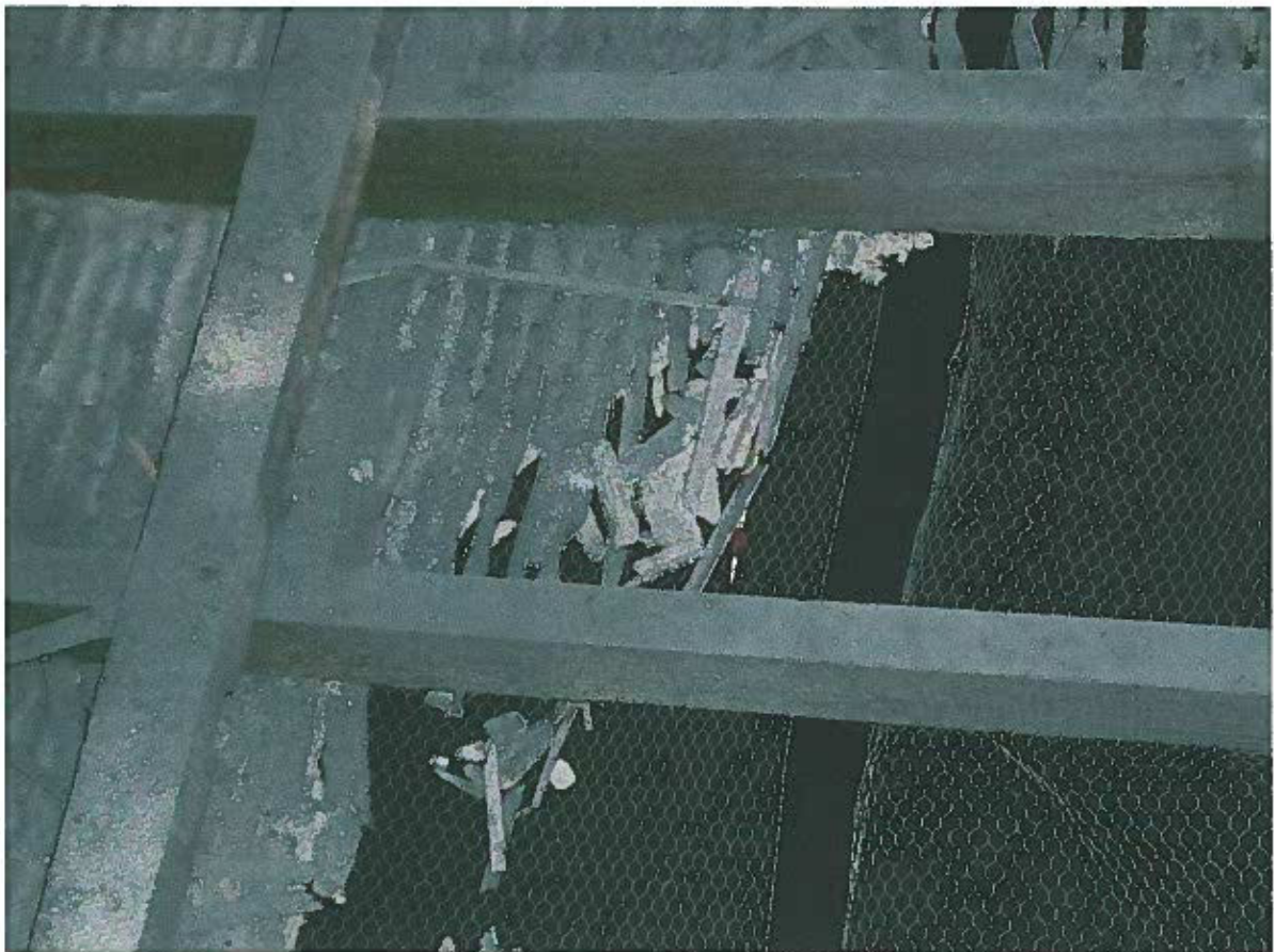
Picture 6 – Failure to ceiling plaster & mesh chicken wire
